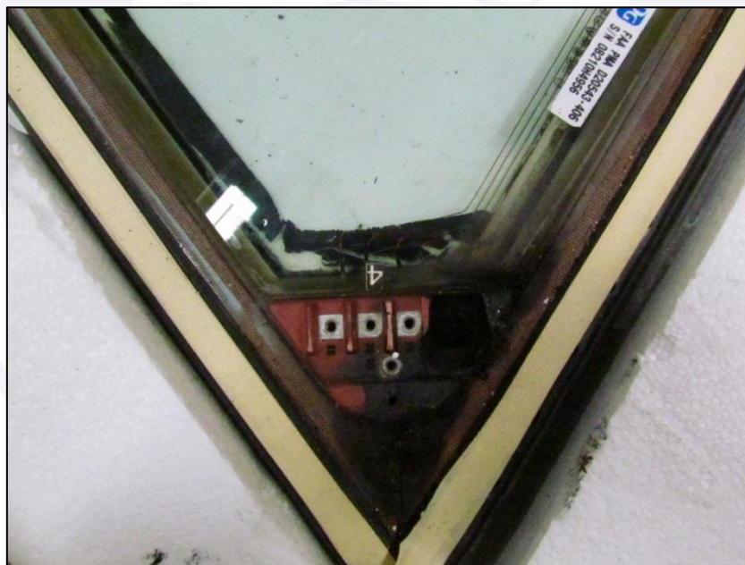
Figure 4 - Windshield: general aspect of the failure.
