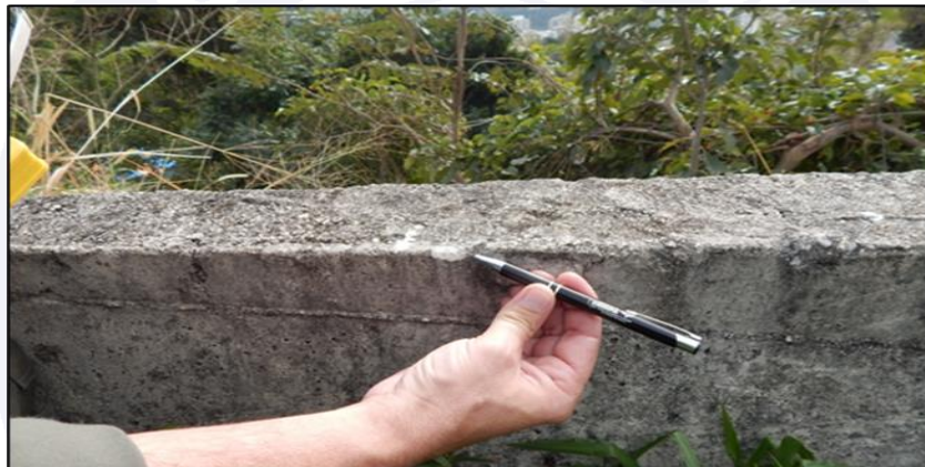
Figure 5 - Point of impact of the tail rotor against the wall.
