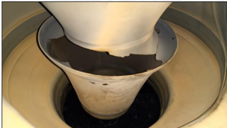
Figure 10 - Internal damage with loss of material in the Exhaust Duct.
