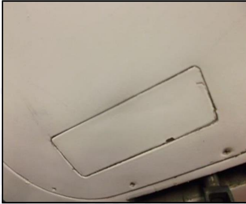
Figure 4 - External view of the fully closed small flap, after manual activation.
