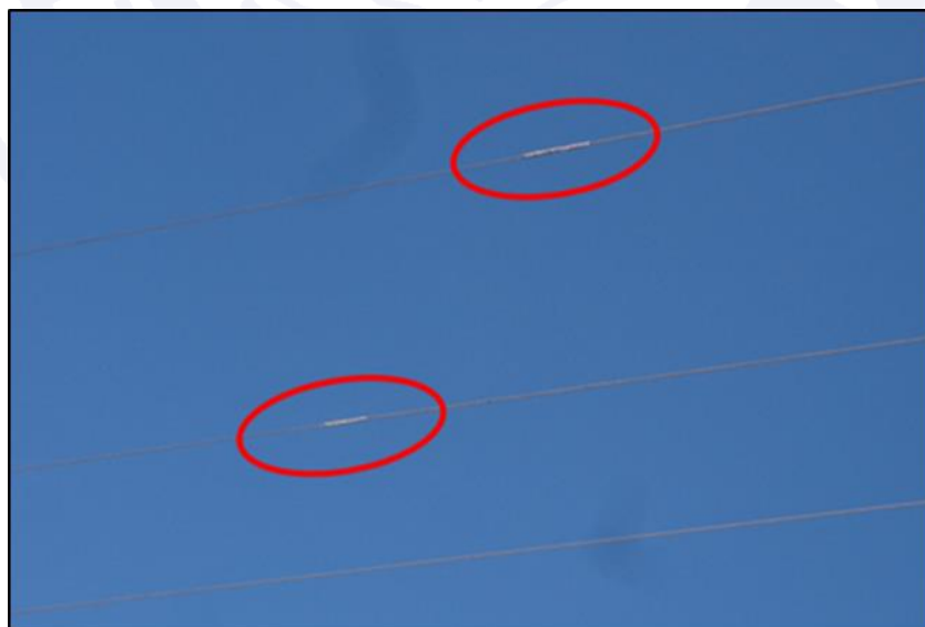
Figure 1 – Low-voltage network, repaired after the occurrence.
