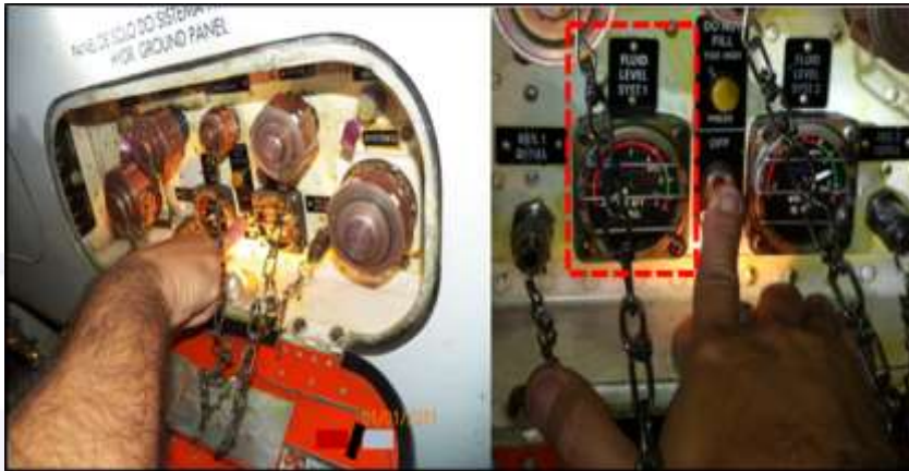
Figure 13 - Hydraulic ground panel and fluid amount detail in system 1.
