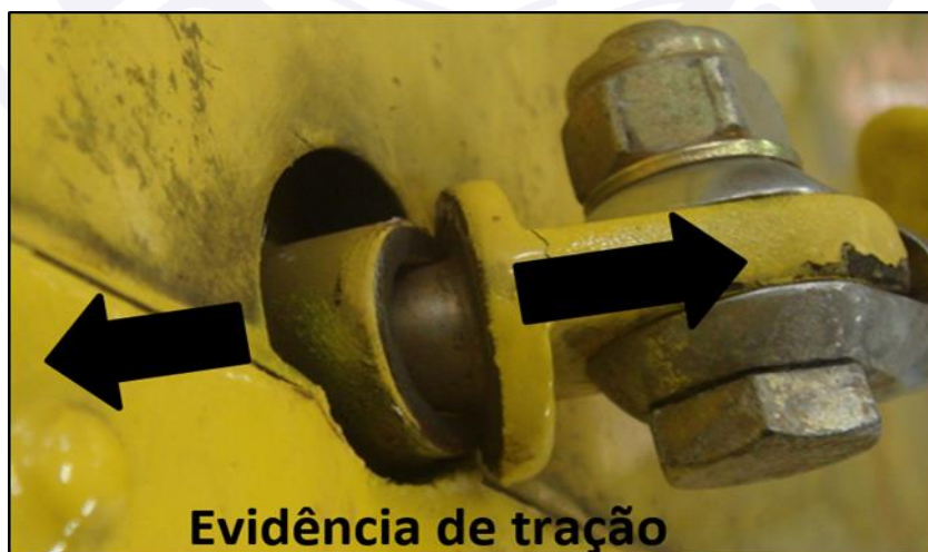
Figure 7 - Fastening of the brace strut with characteristic of overload and tensile deformation (detail of Figure 6).
