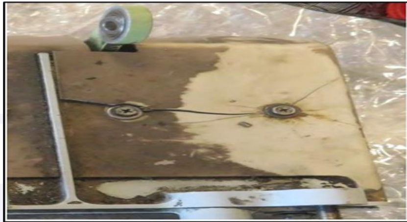
Figure 29 - Damage to the Microswitch Box protection cover.
