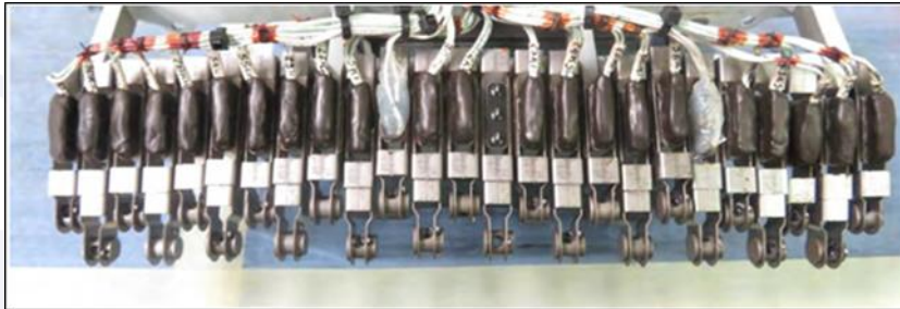
Figure 38 - Microswitches installed in the Microswitch Box, PN 11S76180650-010, SN 0199.
