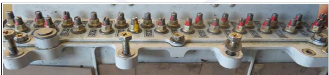
Figure 28 - Misalignment between the adhesive markings on the Microswitches screws and nuts.
