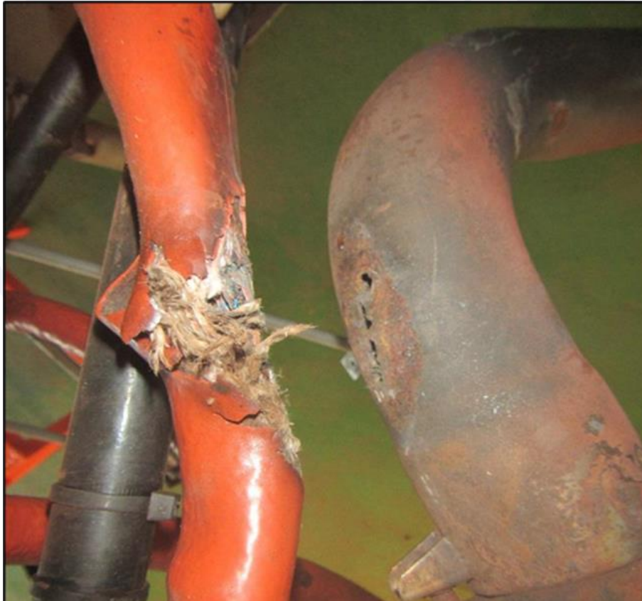
Figure 4 - Damage generated in electrical cabling and exhaust.
