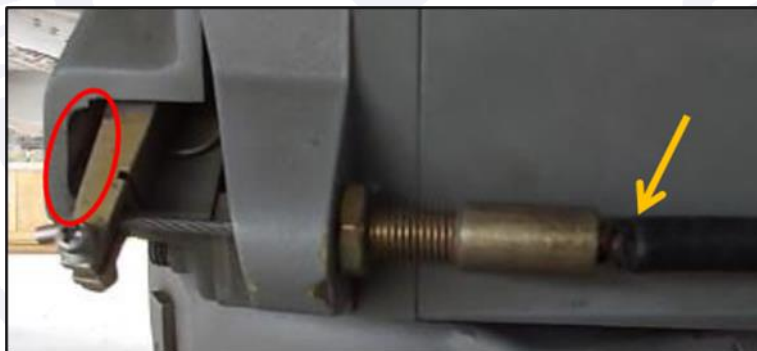
Figure 5 - The red circle shows the clearance of approximately 4 mm between the lever and the housing unit. The yellow arrow shows frayed mechanical drive cable conduit (PN 704A31-813009).
