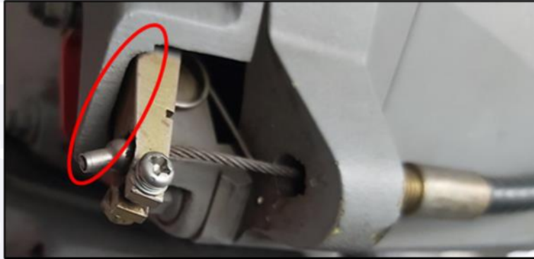
Figure 4 - The red circle shows that there was no clearance adjustment as required on the mechanical drive lever.
