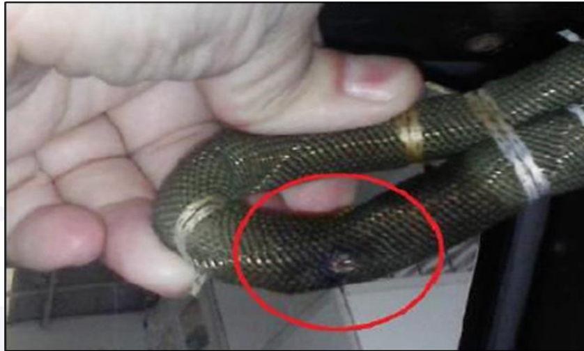
Figure 2 - Overheating marks and hole in the wiring.
