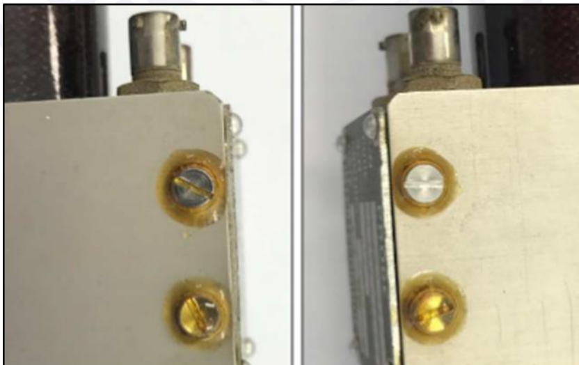
Fig. 17 - Varnish on the screws of the electrical box of P/N 768-100 S/N 516 fuel probe. Source: SAFRAN Investigation Report.
