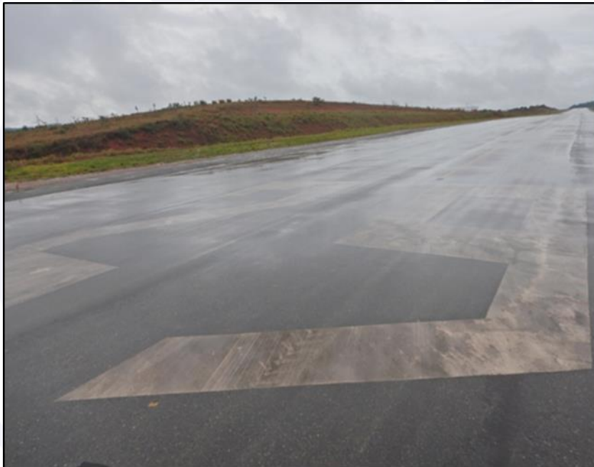
Figure 4 –Threshold 29 of SSDK: wet and mirrored surface after rainfall.
