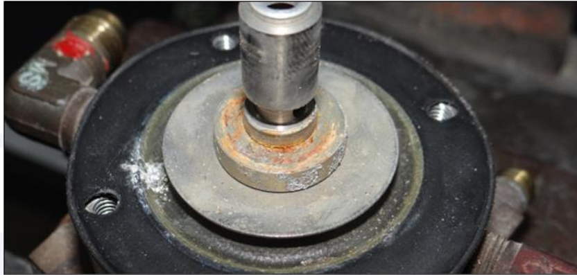
Figure 11 - View of the diaphragm piston stuck by corrosion.
