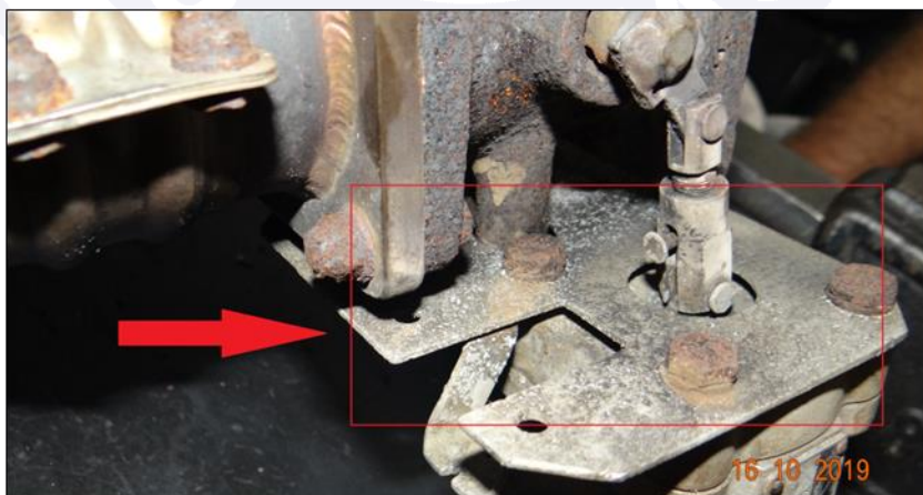
Figure 13 - Evidence of the actuator affected by the leakage of exhaust gases from the throttle body.
