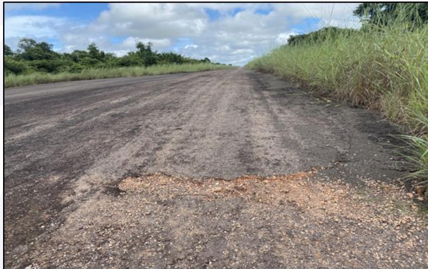
Figure 5 - Asphalt runway with loose rocks.
