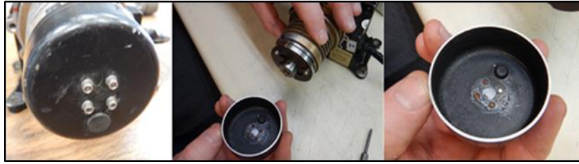
Figure 20 - Cover without the braking on the screws and detail of the debris.
