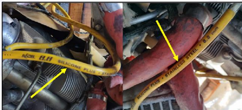
Figure 9 – Spark-plug cables used in the aircraft engine.
