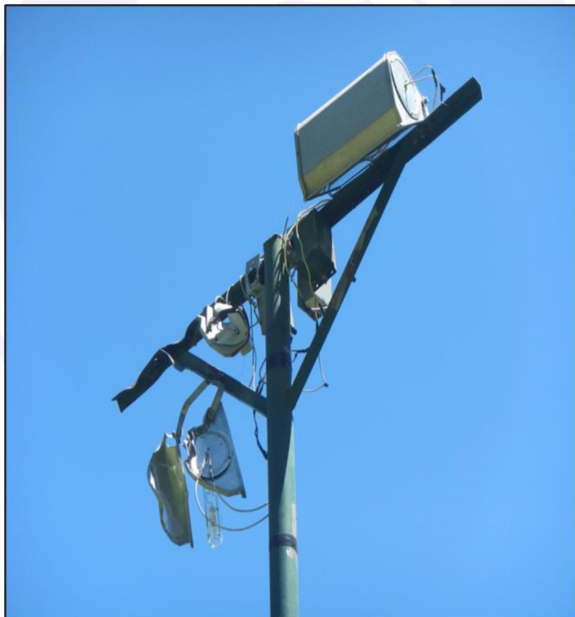
Figure 4 - Detail of the damage to the light pole that was hit.
