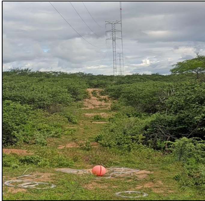
Figure 35 – Aircraft warning sphere nº 1 on the ground, due to breakage of the lightning-rod cable of the 230-kV LT.
