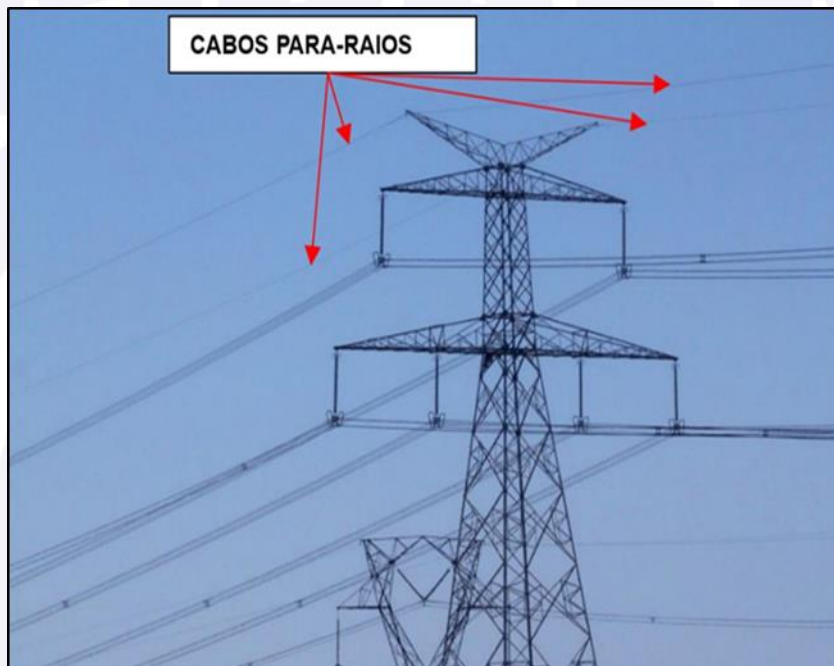
Figure 13 - Illustrative image of lightning-rod cables on the top of a LT.
