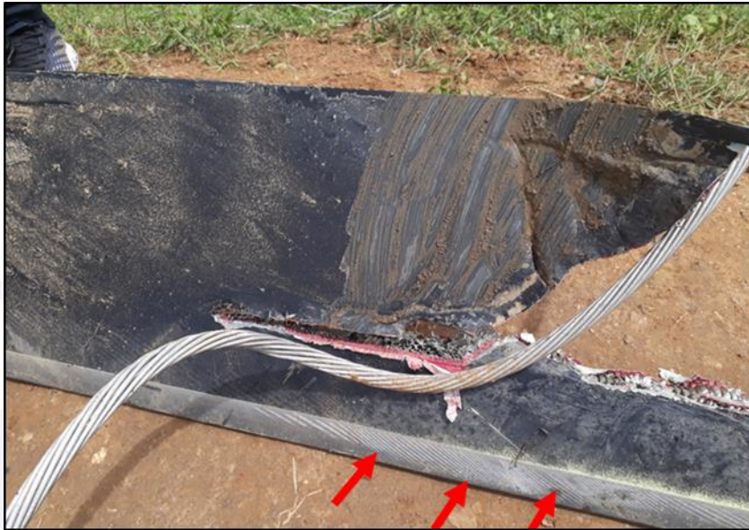
Figure 18 – Contact marks (grooves) between the lightning-rod cable and the leading edge of one of the main rotor blades.
