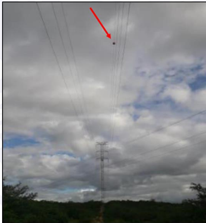
Figure 36 - Warning sphere nº 2 of the 230-kV LT
