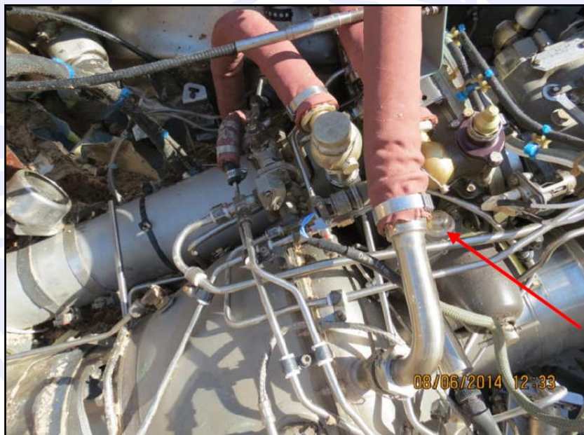
Figure 33 – Pre-blockage Indicator of the engine oil filter (not popped-out).
