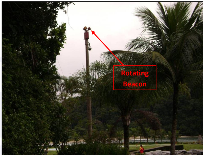
Figure 3 - Tower (Rotating Beacon) installed close to the Helipad.
