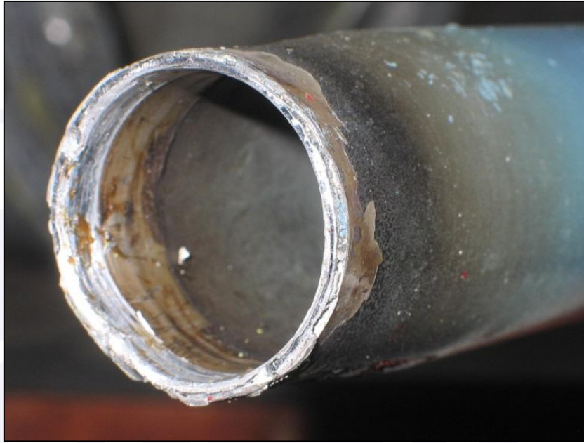
Figure 15 – End of long shaft broken at the point of connection with the short shaft.
