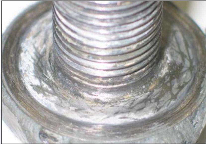
Figure 9 – Mark of circular friction on the lower part of the fastening-bolt head.
