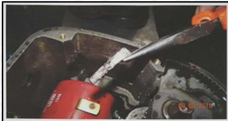
Figure 8 - View of one loose coil lock inside the left magneto.
