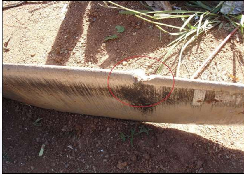
Figure 4 - Impact point of the propeller against the power grid (lightning arrester).
