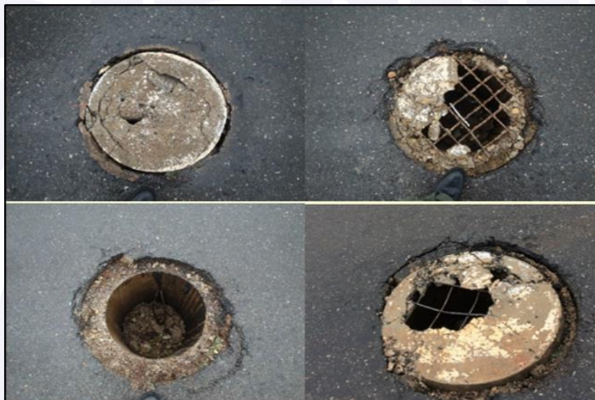
Figure 9 - Damaged electrical passage boxes.
