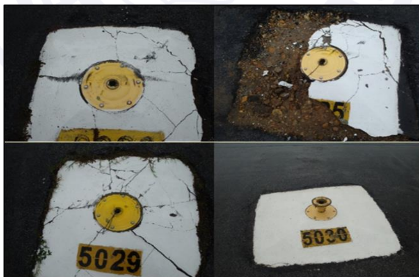
Figure 7 - Damage to the vertical markings of runway 11L.
