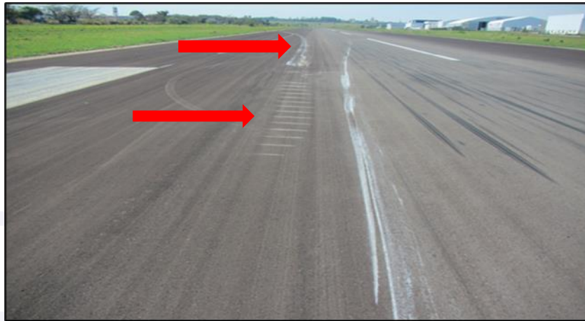
Figure 6 - Marks left by the contact of the rudder, propeller, engine hood, spinner and right wing with the runway.
