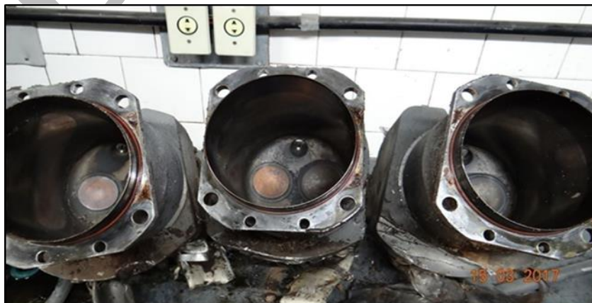
15 16 Figure 25 - View of cylinders 4, 5 and 6, without operational damage. 17
