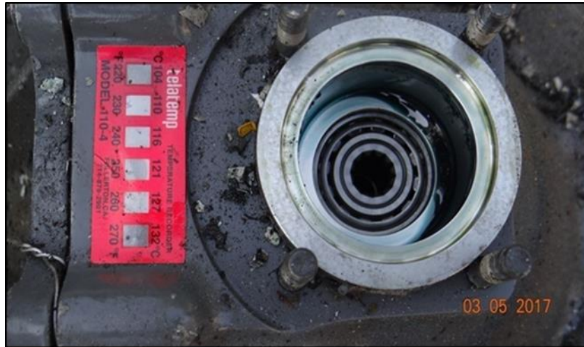
5 6 Figure 38 - Housing of the hydraulic pump in the gearbox.
