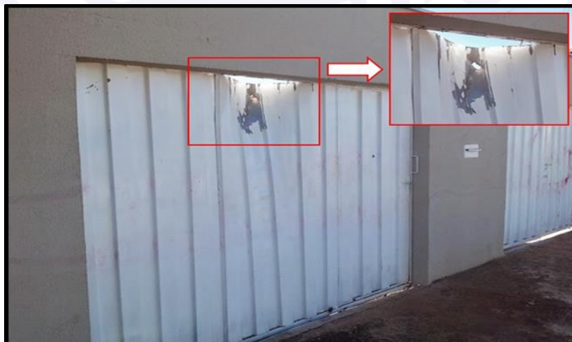
Figure 4 - Damage to the gate of a residence.
