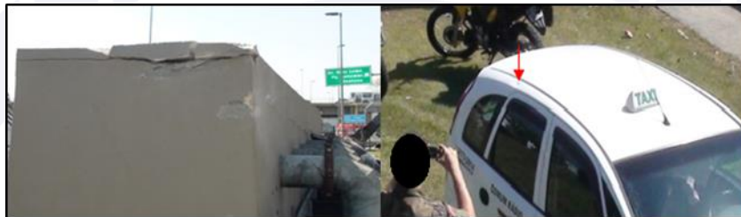
Figure 3 - Damages to the concrete wall and the car.
