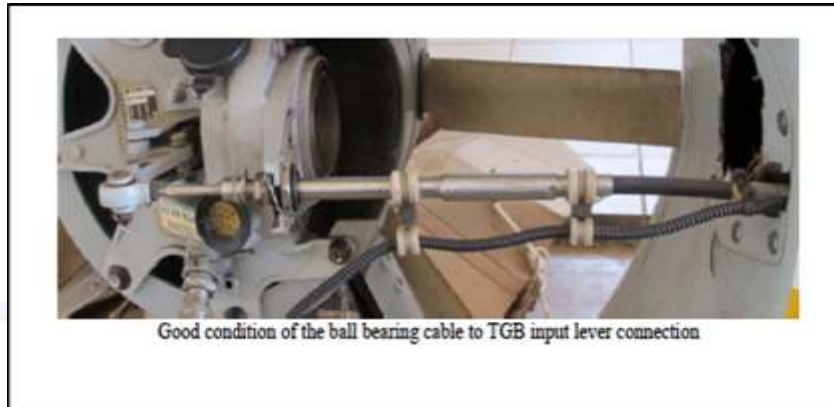
Figure 35 – Good condition of the connection of the teleflex cable to the TGB.
