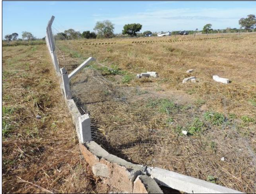
Figure 3 - Wire fence with pillars and concrete foundation overturned by the aircraft.
