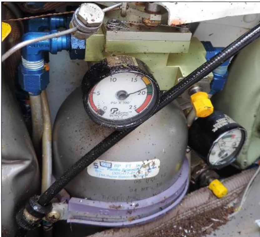
Figure 13 - Nitrogen accumulator of the emergency brake system (green band from 1,800 to 2,050psi)
