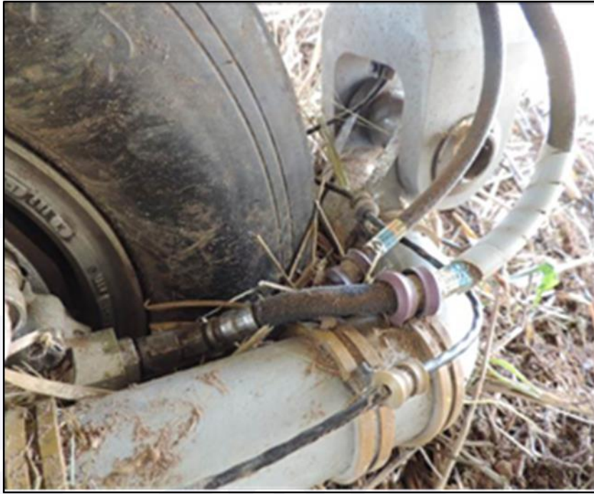
Figure 12 - Hydraulic power line and nitrogen vent line of the brake system.
